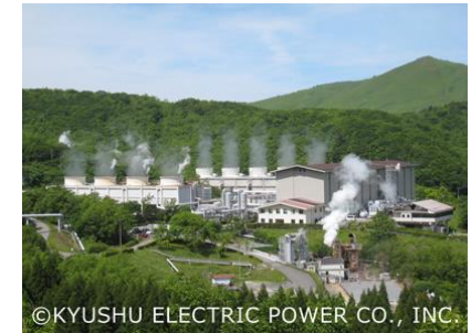
Hatchobaru Geothermal Power Station
